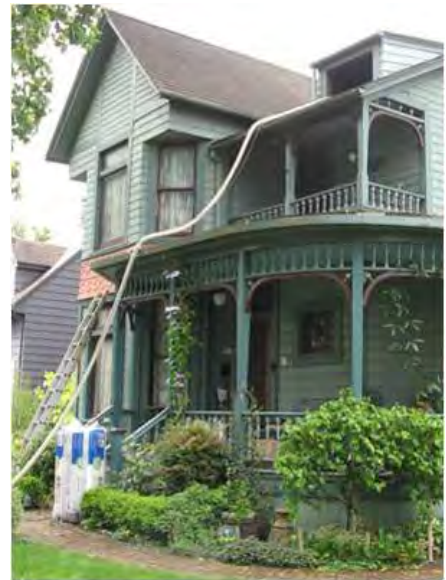
A Department of Energy-funded project in Washington provides insulation for this historic home. (photo courtesy DOE)
