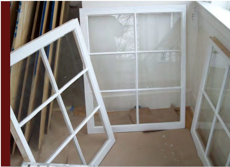
Photos: Above, replacement window installation underway; Right, a worker repairs, abates historic frames on a house in Fort Belvoir Historic District. (photos courtesy U.S.Army)
