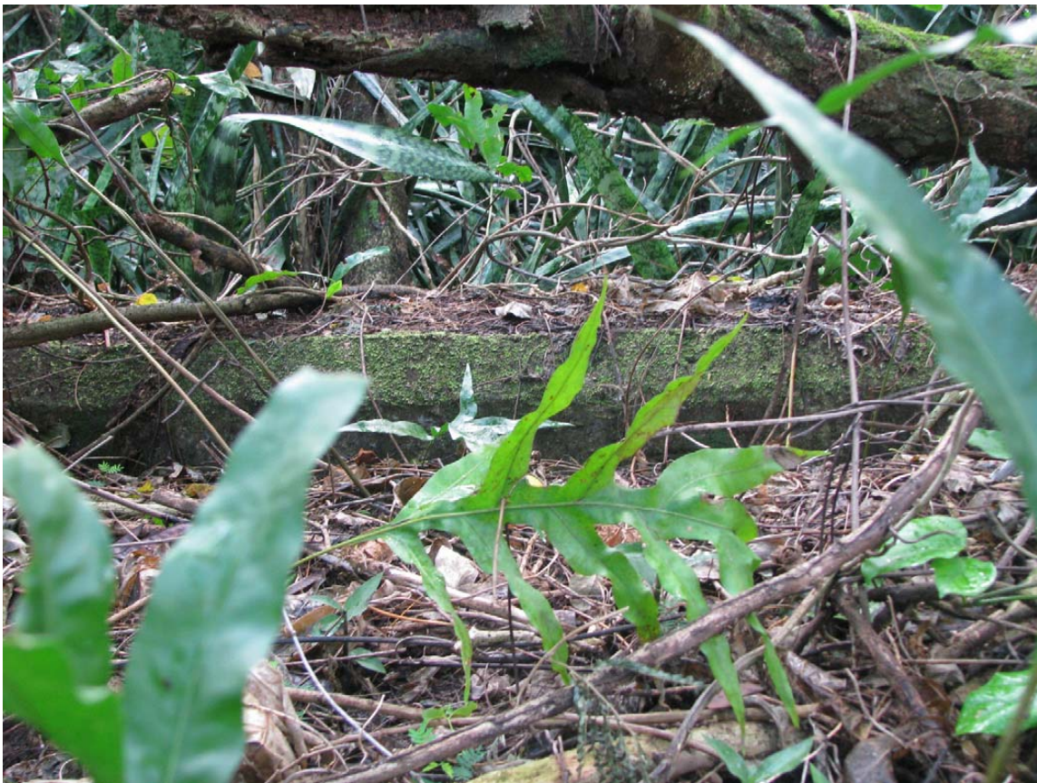
Example of a Quonset hut foundation covered with vegetation, at the site of the 121 st NCB Group Service Area ( CLR , 3-44).
