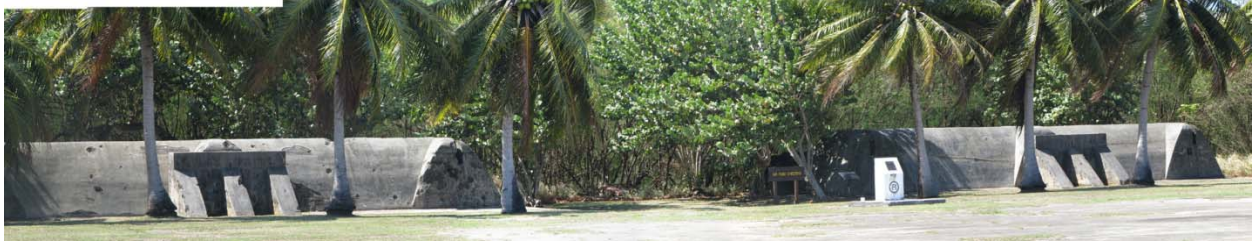
Japanese air raid shelters on the Japanese air apron. Character defining strafe marks are visible ( CLR , 3-40).
