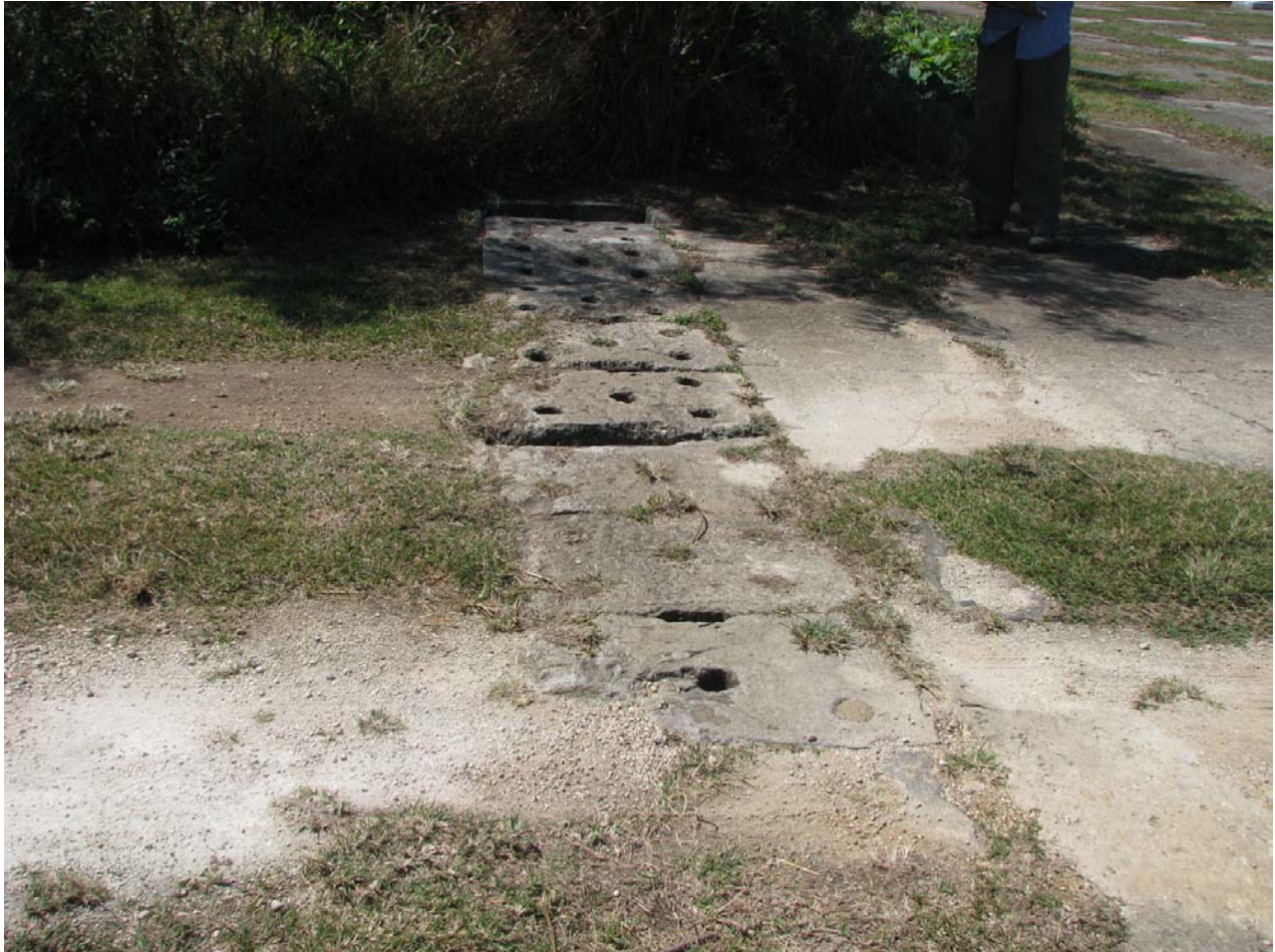
Character defining concrete covers on Japanese drainage canal, on the edge of the Japanese air apron (CLR, 3-43).
