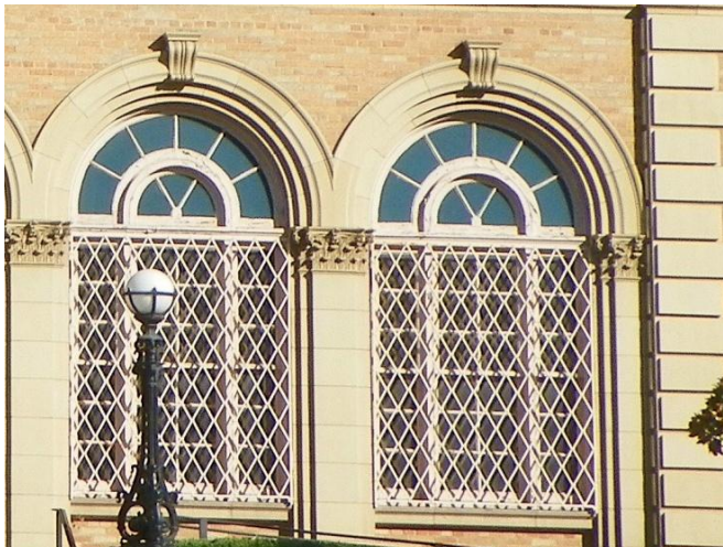
Pair of large tripartite, double-hung, wood windows (6/6, central window flanked by 3/3 windows on each side). Semicircular fanlights above each window, terra cotta sill below. Covered with decorative wrought-iron grilles. Grilles to be removed, windows to be restored.
