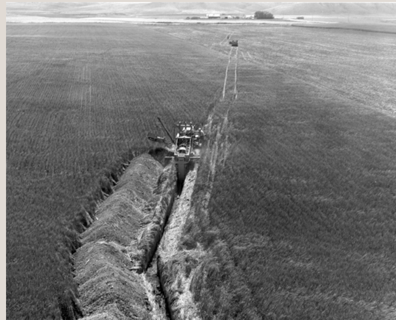
Construction crews trenched miles of utility corridors in the 1960s during the original construction of the Minuteman missile fields, before passage of the NHPA and NEPA. (USAF)
