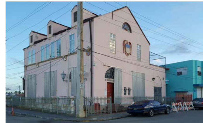
The U.S. Custom House in Fajardo, PR, played a vital role in Puerto Rico's transition from a Spanish to U.S. colony in the 1890s. The Custom House was severely damaged by Hurricane Maria in 2017 (left), but was extensively repaired and renovated during the reporting period (right). (CBP)
