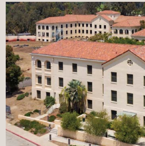
Buildings 205 and 208 of the VA’s Greater Los Angeles Healthcare System West LA Campus under construction (VA)
