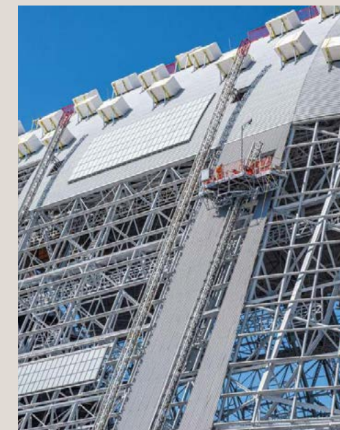
The re-cladding of Hangar 1 began in mid-2022 and is currently in progress. (Planetary Ventures)
