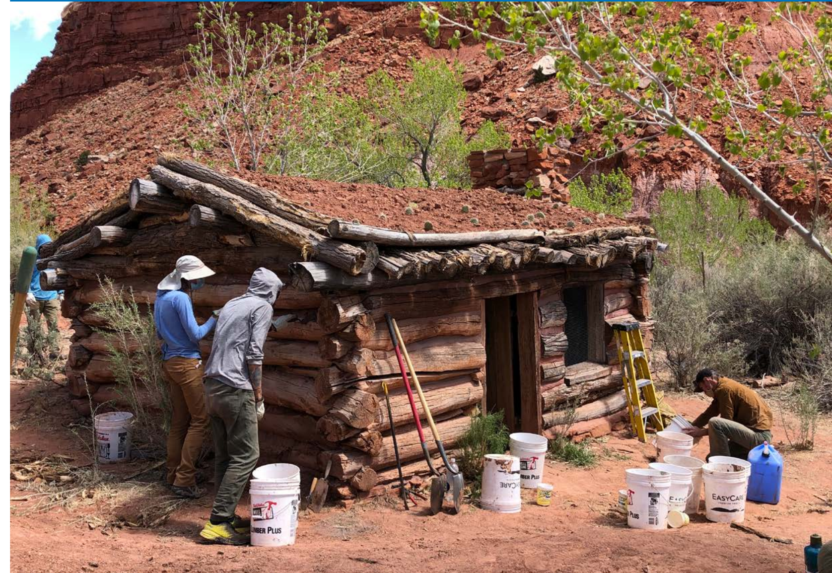
Southern Utah Wilderness Alliance volunteers work on restoring the roofing and chinking of the historic Watson Cabin within the Paria River District, UT. (Valerie Russell/BLM)
