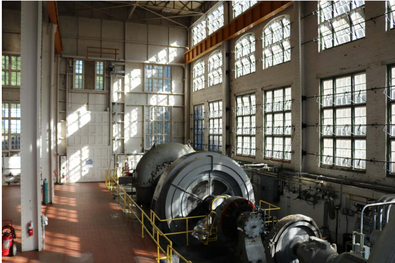
TVA recently focused on the maintenance and rehabilitation of the three plants of the Ocoee Plant group in Polk County, TN. Large banks of wood windows have suffered damage due to increased humidity and extreme temperatures. (TVA)
