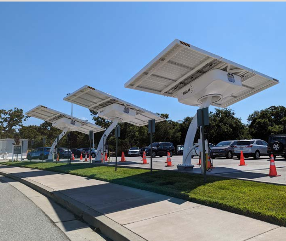
The EVSE exemption has allowed VA to focus on clean energy and infrastructure within Veterans Health Administration facilities. About 140 EVSE units have already been installed, including EV charging stations pictured here within the Palo Alto VAMC. (Angela McArdle/VA)
