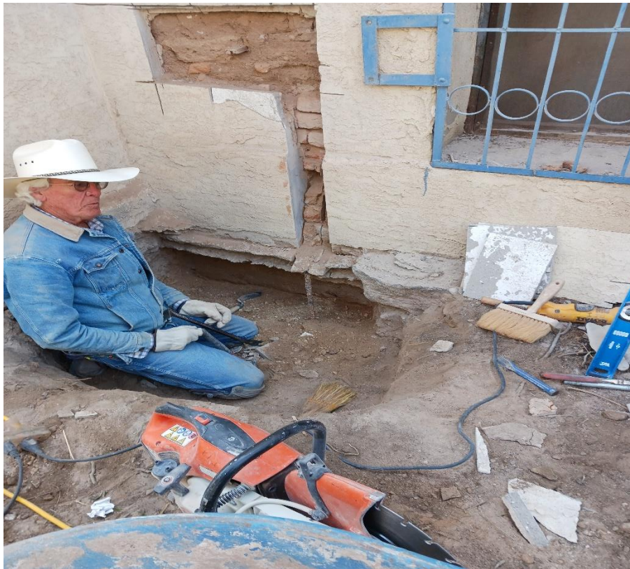
Figure 9: Adobe Restoration expert Pat Taylor working on examining the original adobe wall behind modern concrete, brick, and chicken wire cover. This project was to examine the effects of moisture on the mid 1800s building and what can be done for restoration and preservation. This is next to the USIBWC American Canal, U.S. – Mexico International Boundary and part of old Fort Bliss from the 1870s.
