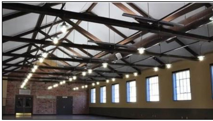
Interior of the historic pool house at Camp Dodge Joint Maneuver Training Center.
