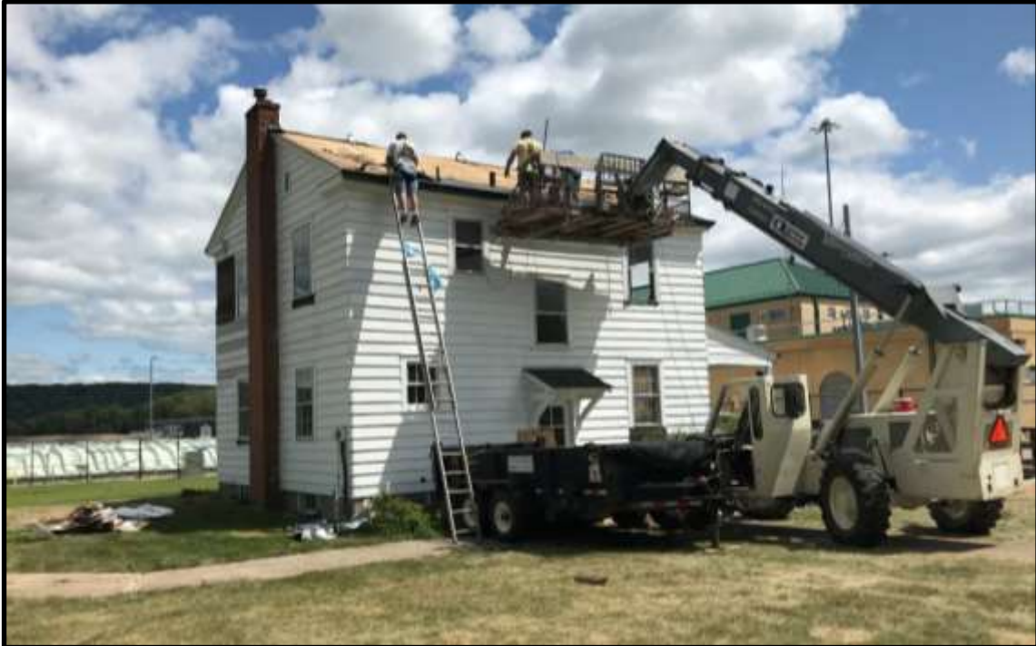
Figure 8: Rehabilitation of the Lock and Dam 10 Lockmaster house for use as a museum.
