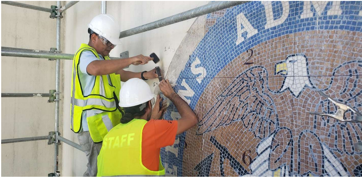
Figure 5 (below): An artisan removes the Veterans Administration mosaic from Building 1 of the San Juan VAMC. It will be reinstalled at the pedestrian level on campus.
