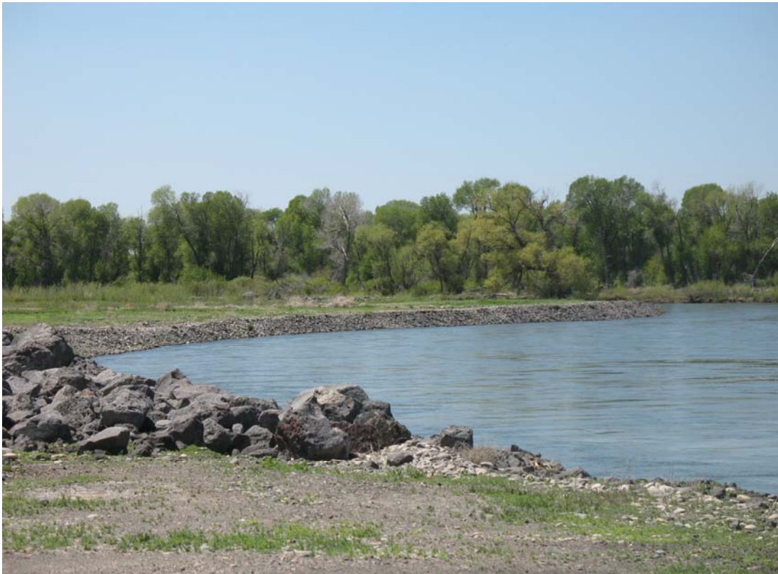
Figure 2. View of rock armoring installed to stabilize and protect eroding banks upstream of the Fort Hall NHL, Idaho
