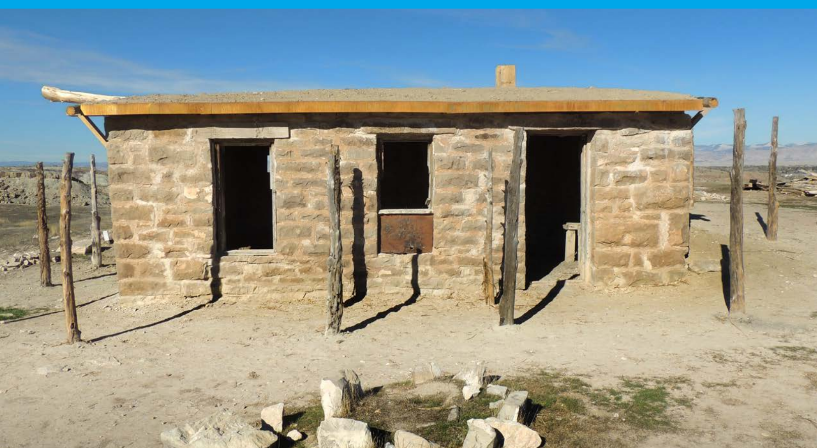
Completed rehabilitation work at Skinner Cabin, McClinnis Canyon National Conservation Area, CO (BLM/Natasha Krasnow)
