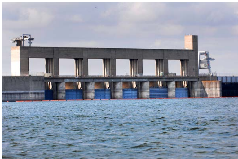
Falcon Dam is the lowermost major multipurpose international dam and reservoir on the Rio Grande. (USIBWC)
